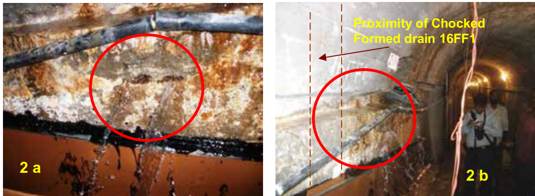
Picture 2 Photograph showing leakage at ch.434 m in intermediate drainage gallery; a. leakage in block joint 15/16; b. Photograph showing the proximity of chocked formed drain to the leakage point in block joint 15/16
